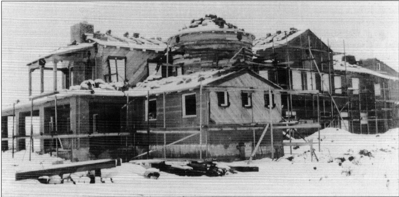
The Red House "Mansion" under construction by Andy Williams during a snow in 1930.
