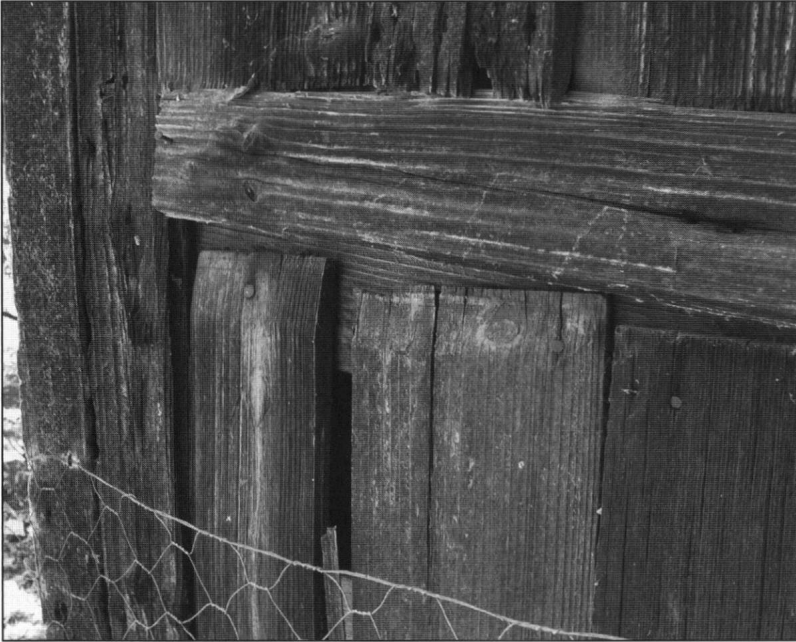
Shrinkage of the fitted joints required supplemental nails, not intended as an original requirement.
