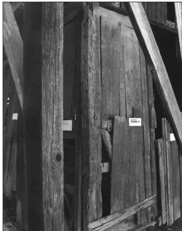
Extreme weatherization and shrinkage of the wood had left much of the original structure vulnerable to time.
