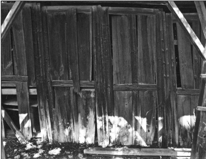
Severe shrinkage of the wall panels had rendered the sides no longer tight and well fitted. Nails were required to hold the structure together.
