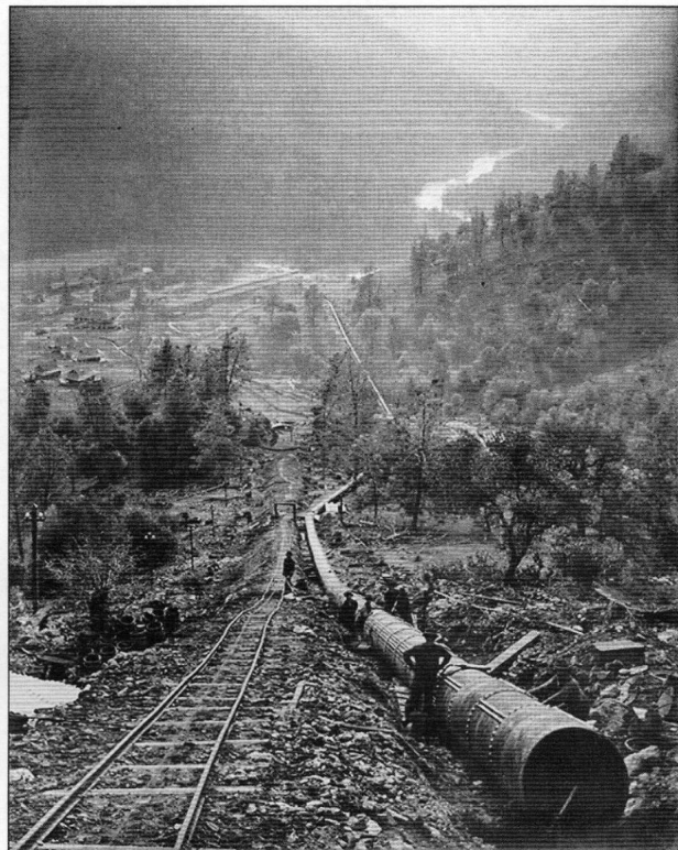
Electra Powerhouse Penstock under construction. The penstock, with a vertical drop of 1220 feet, carried water to power the turbines.
