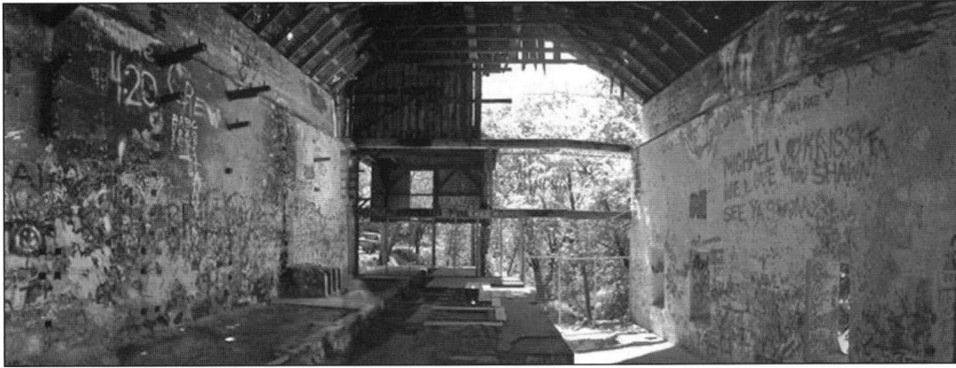
Little was left of the downstream wall of the building when Martin Huberty purchased the powerhouse.
