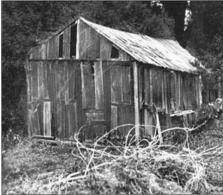
Eighty years of neglect was becoming apparent on the Chinese building in this 1932 photo.
